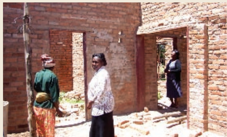
The women molded the bricks at home and carried it to the site they negotiated with the council
